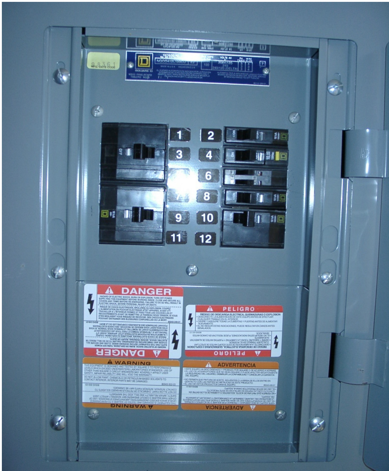
Circuit Breaker Panel (CL)
