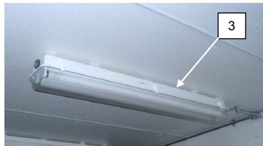
Containerized Latrine System
